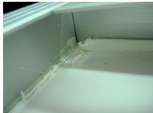
Figure 6: Non uniform sealant in the back sheet. It can produce inclusion of moisture and dielectric problems.
